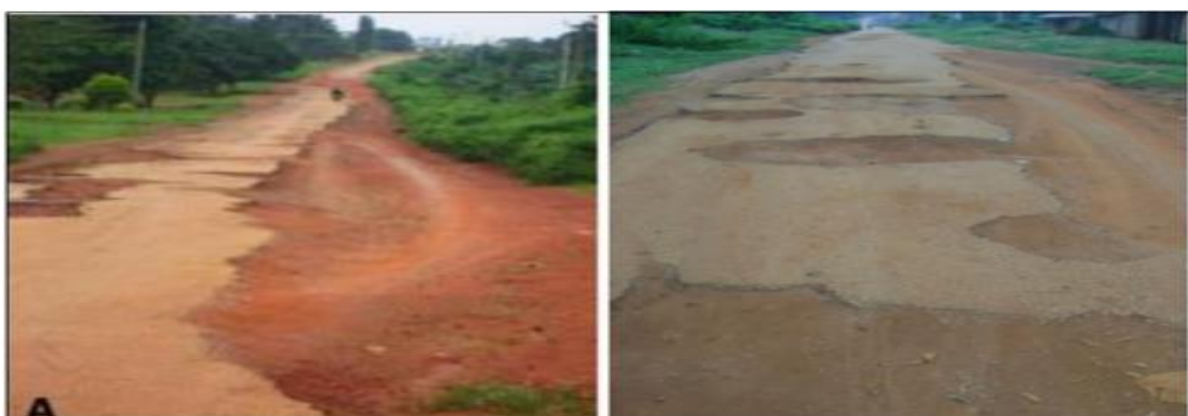
Fig.2: Failure portions of the Road segment identified at Federal College of Education (Technical), Asaba, Delta State.
